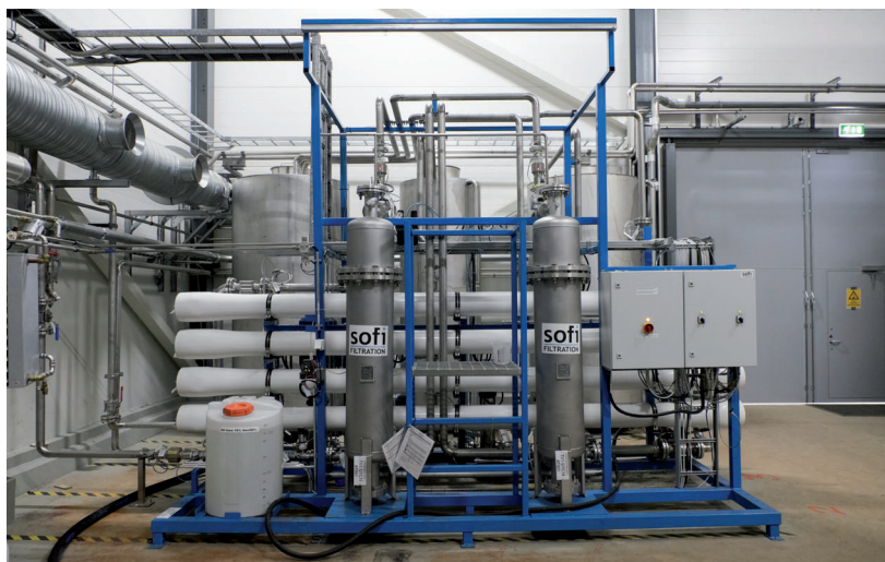
Sofi Filtration's water treatment system.
