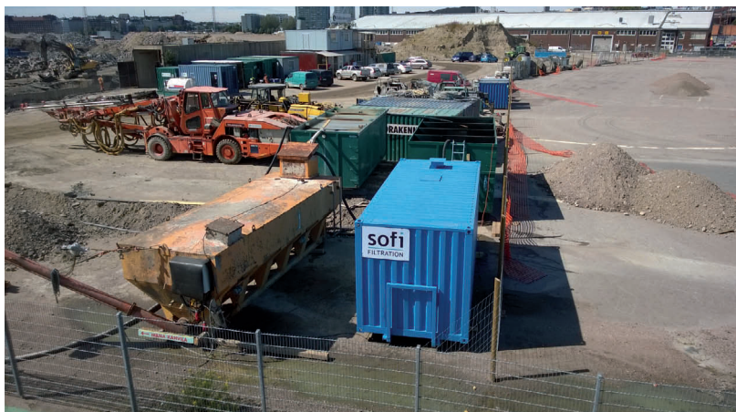
Figure 1: The Sofi Filtration system on-site at a tunneling operation in Helsinki.
